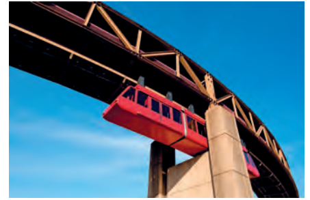
Photo 1.2 This bridge truss consists of two-force members that may be in tension or in compression. ©Natalia Bratslavsky/Shutterstock
